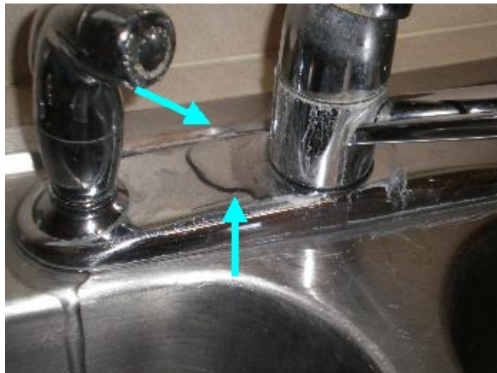
Faucet leaks while operating
