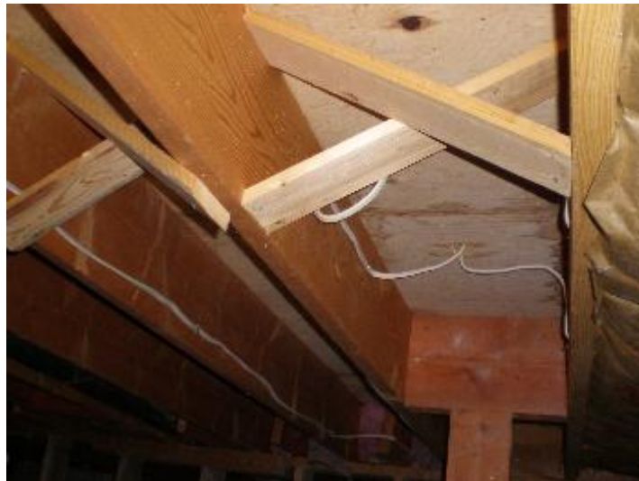
Only partial insulation installed, (rolls of insulation present)
