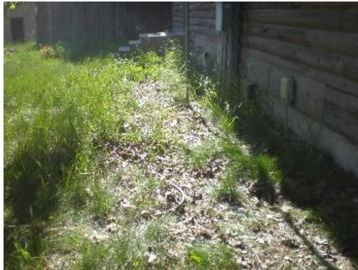
Flat or slopes towards structure in some areas
