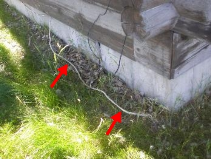
exposed unanchored romex wiring, (evidence of broken insulation)
