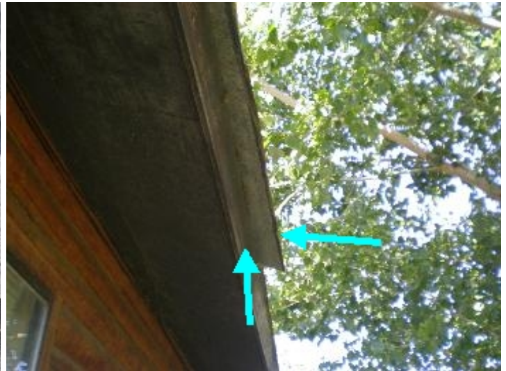
Metal used as starter course loose, needs reattached
