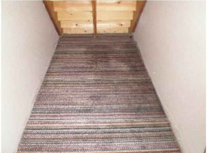
Evidence of water/moisture infiltration from mechanical room (possible micro-bio-growth present, Consult qualified professional)
