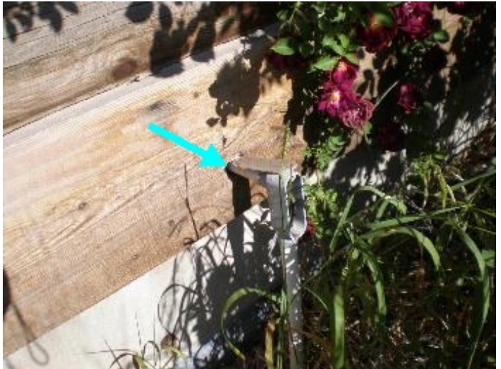
Exterior penetrations not sealed to improve caulk/reseal to prevent moisture/insect penetration
