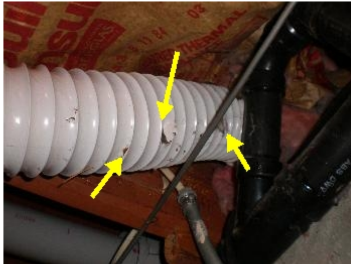
damaged vent pipe
