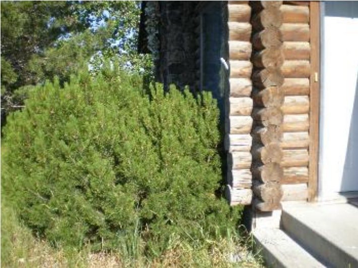
Trees/shrubs overgrown/contact with structure in some areas (recommend trim to prevent damage)
