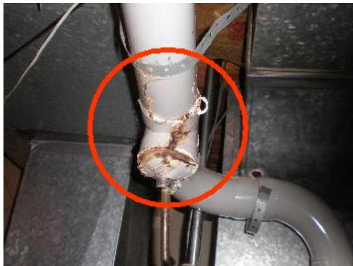
Damaged vent pipe (evidence of unsuccessful repairs)
