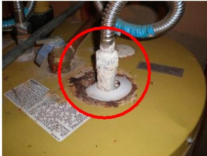
corrosion present (possible di- electrical reaction) dissimilar metals
