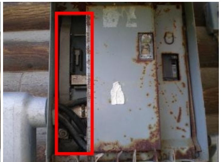
missing inside cover
