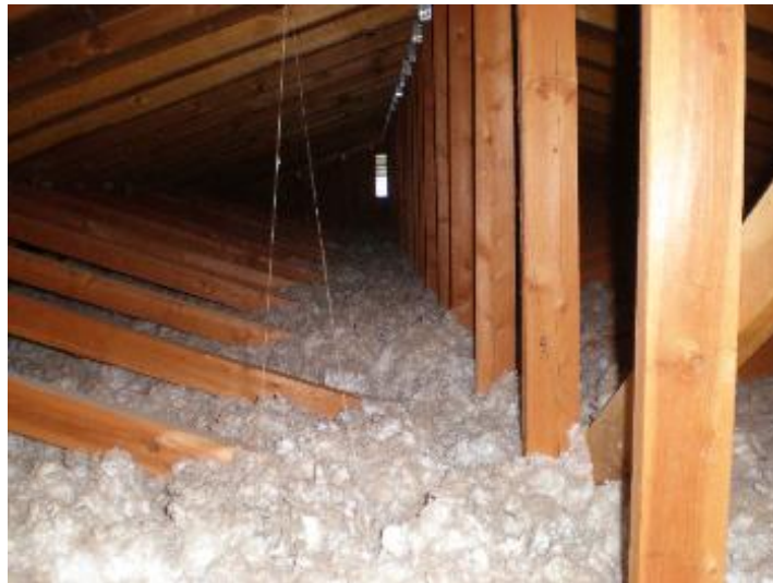
recommend adding additional vents (to improve only, adds life to roof covering)
