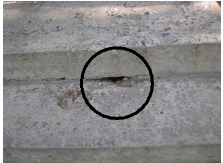
Rear concrete steps have hole present, (recommend seal to prevent moisture/insect intrusion)
