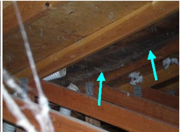
Evidence of possible micro-bio-growth (due to improper ventilation)
