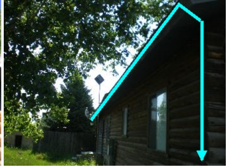
Recommend to improve; install rain gutters & downspouts
