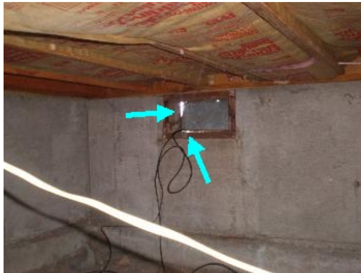
Vents not properly secured, Gaps present due to cable installation allowing insect intrusion, recommend seal/re-attach
