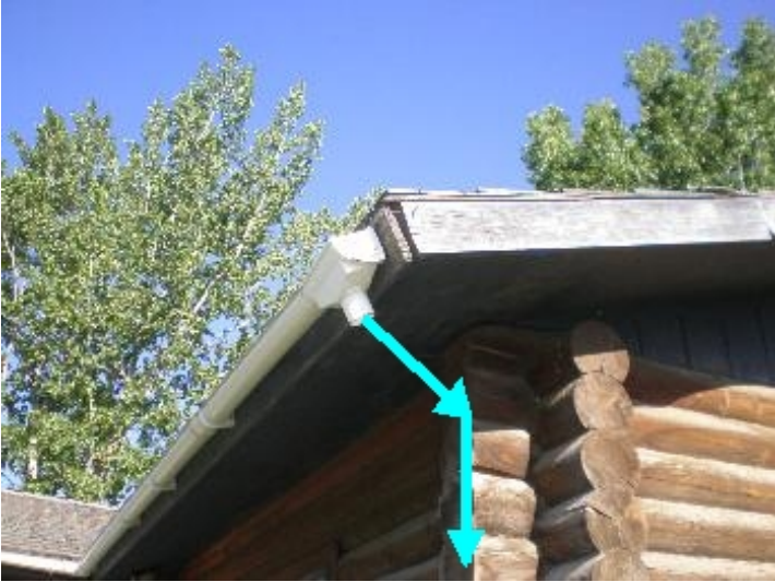
missing down spouts
