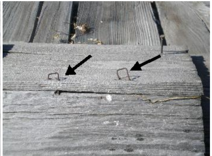
Ridge cap nails/staples backing out
