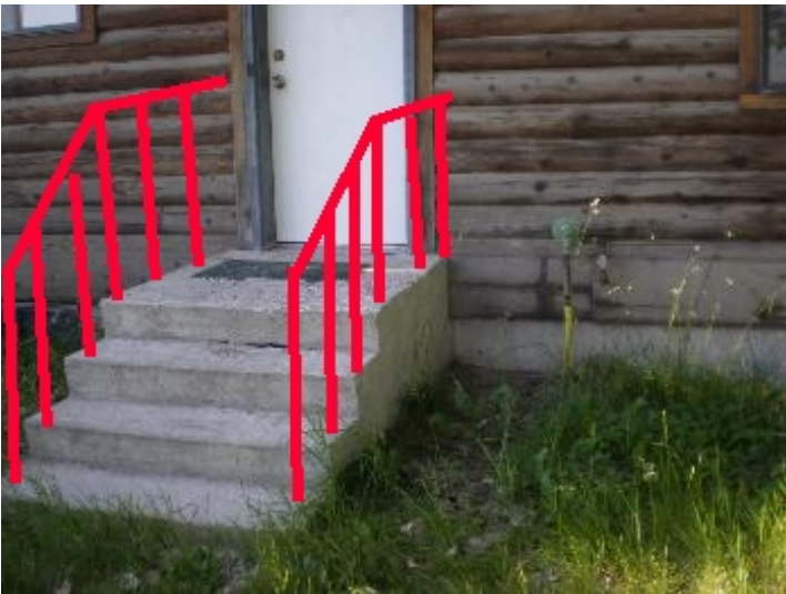
No hand railing (4 or more steps require a handrail)
