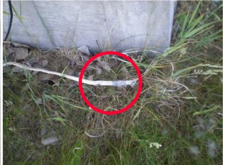
exposed romex wiring, (evidence of broken insulation)
