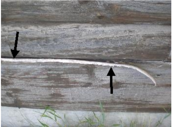
Chinking missing/deteriorating in some areas
