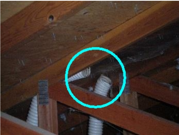
Bath exhaust fan does not vent to the exterior (causes moisture build up/possible dry rot)
