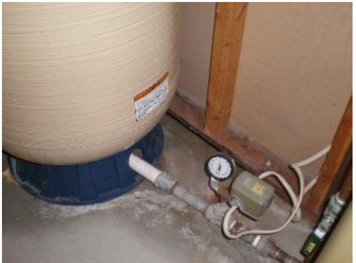
Evidence of current leak at pressure tank
