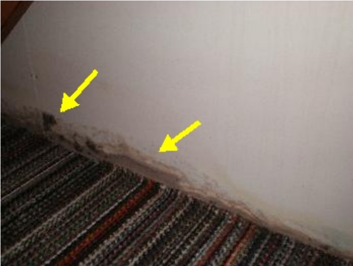
Evidence of water/moisture infiltration from mechanical room (possible micro-bio-growth present, Consult qualified professional)
