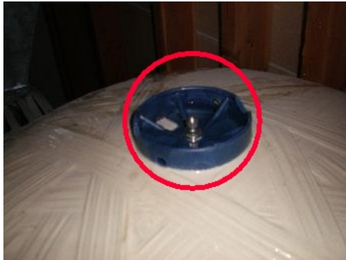
Evidence of standing water at pressure tank relief valve
