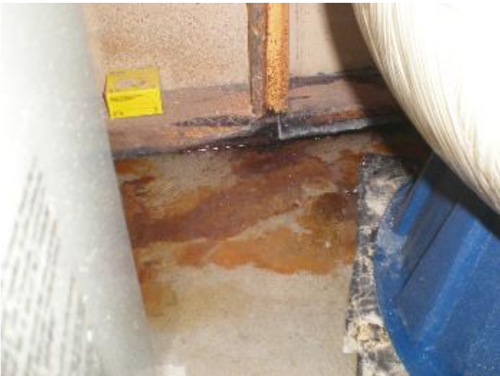
Evidence of current leak at pressure tank
