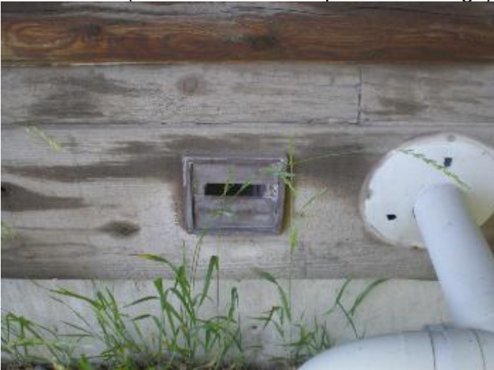
Dryer vent cover damaged/ missing
